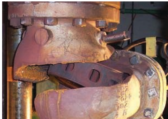
Water hammer can cause catastrophic pipe damage.
