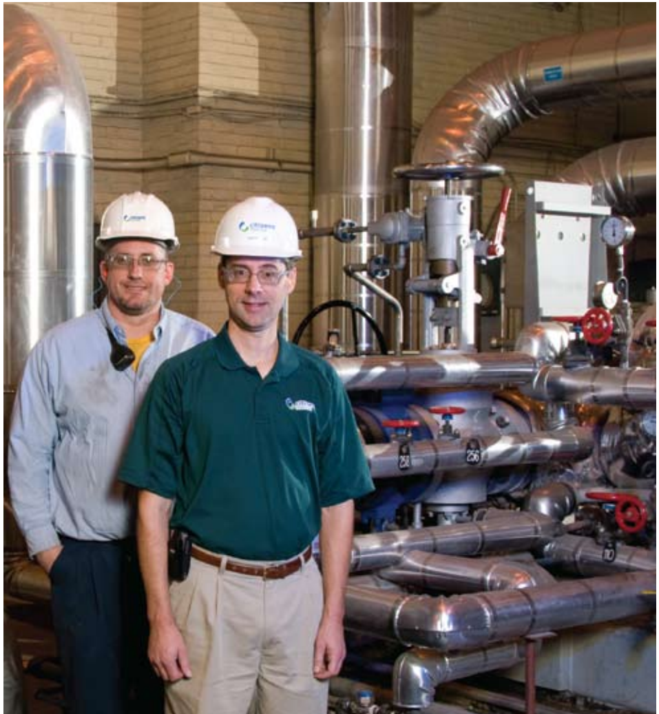
Mike Williams, Operations Auxiliary Operator, and John Havard, Project Manager, ensured the new topping turbines at Perry K provided efficiency improvements to the plant.
