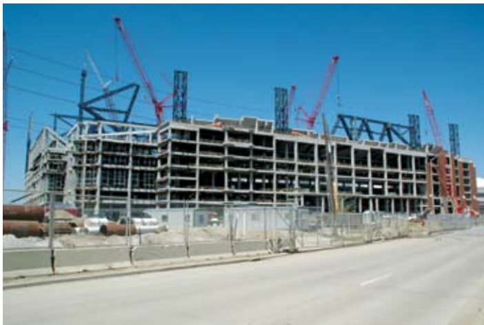
Lucas Oil Stadium is one of the most visible projects in the booming Downtown Indianapolis area. The stadium will use steam and chilled water from Citizens Thermal Energy.
