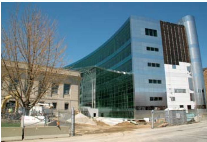
The new Central Library in Downtown Indianapolis is being transformed into a 21 st century learning destination.
