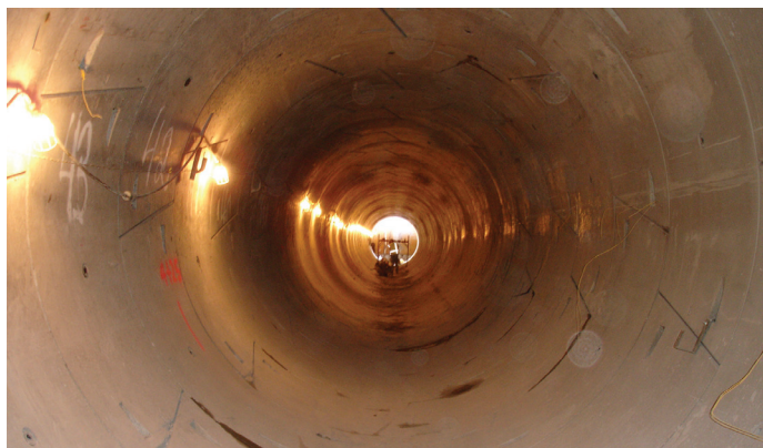
The completed tunnel will be 18 feet in diameter and stretch more than seven miles underground.
