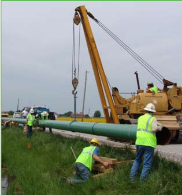
Citizens Gas utilized diverse contractors and suppliers during the construction of the Heartland Gas Pipeline.
